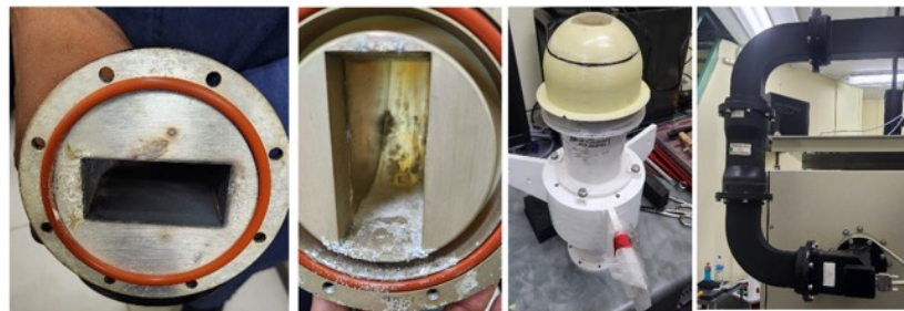
Heavy corrosion on wave guide. New waveguide rotary joint installed. Feed horn changed.
