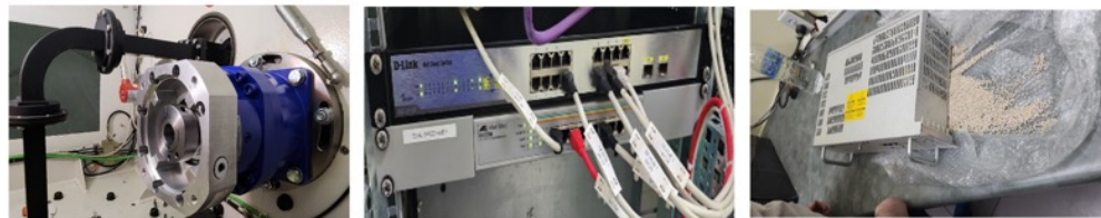
New gearboxes installed. New signal process installed, D-link switch changed. New dehydrator repaired installed
